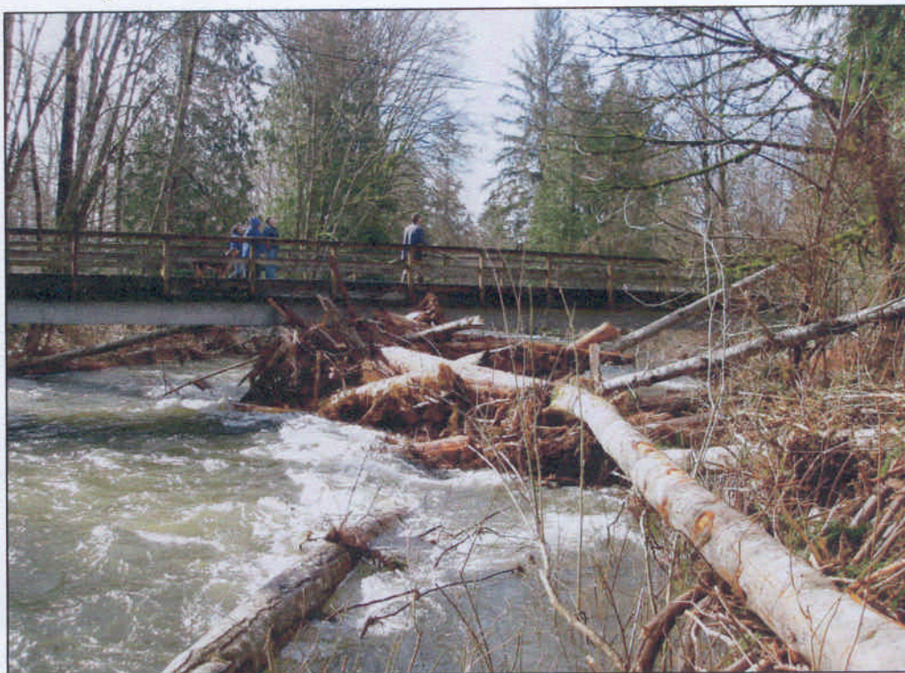
Figure 5: Bridge 2 and the mass of woody debris pushing up against its upstream side.
